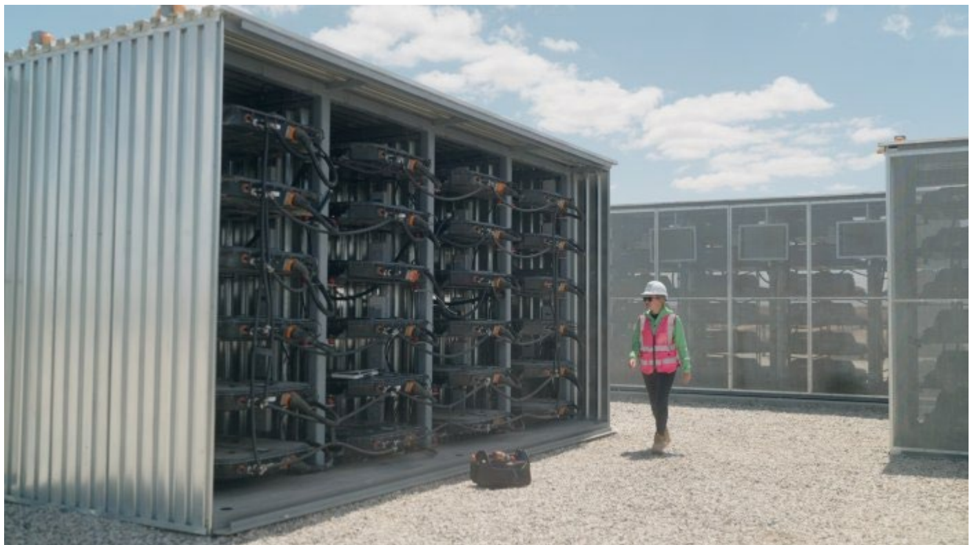
A B2U energy storage system in Lancaster, Calif. PHOTO: AWARDED GOODS
